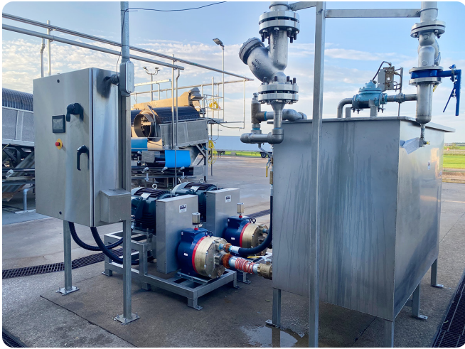
High Pressure Sanitation Systems
