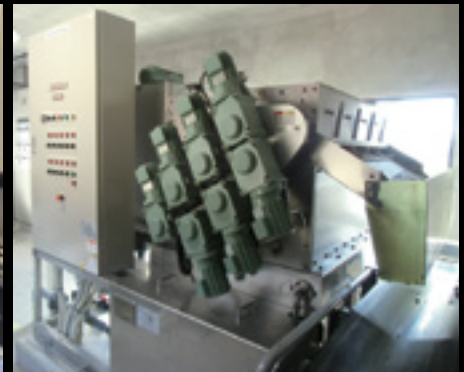
Excess Sludge at Noodle Production Plant (JD-1000)
