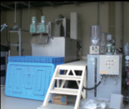
Excess Sludge at Industrial Plant (MDQ-202)
